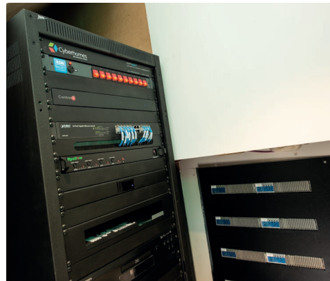
AV racks have plenty of space for the final homeowner to add additional equipment.
